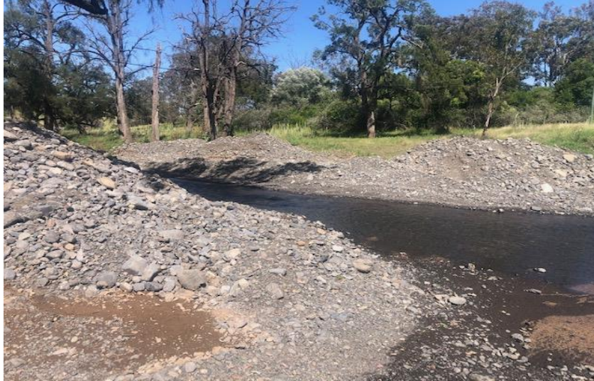
Culvert clearing by LPSC illustrating downstream rockpiles and reinstatement of the original issue.
